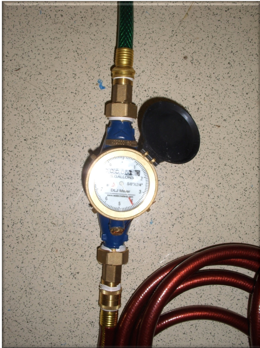
Figure 13: Volumetric Flow Meter (Gal)
